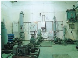
Testing area for Roots Blower
